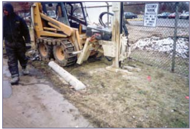
Delivery and injection must conform to the aquifer physical characteristics, which is always defined by our team of hydrogeologists during the investigation phase.
