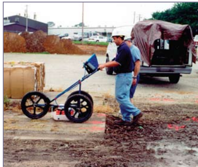
SER 90 , Inc. team using SIR 3000 ground penetrating radar (GPR) to detect buried drums, wastes and other objects.
