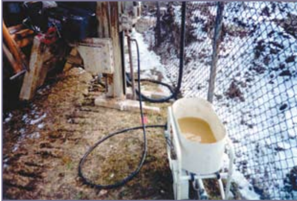
SER 90 , Inc. designed and mass produced bio-augmentation on site for proper Plate Count and a good bioremediation head-start.
