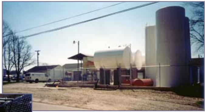
General view of installed SPCC compliance action
